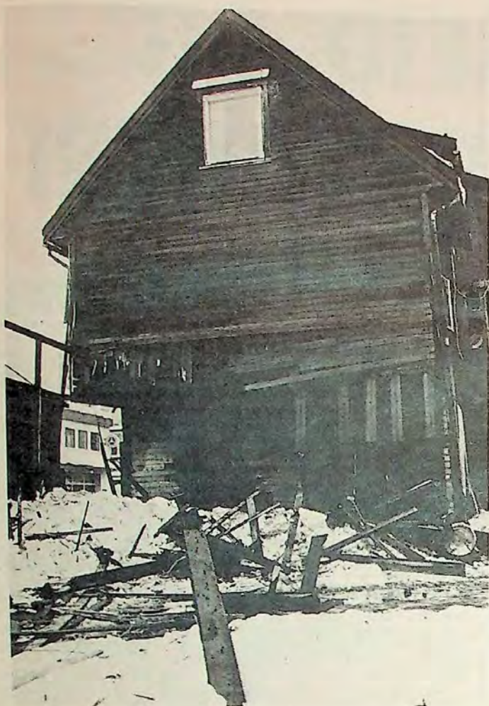
PICTURE: It is pure chance that no one was killed or injured in this building. (Photo: Klassekampen)
